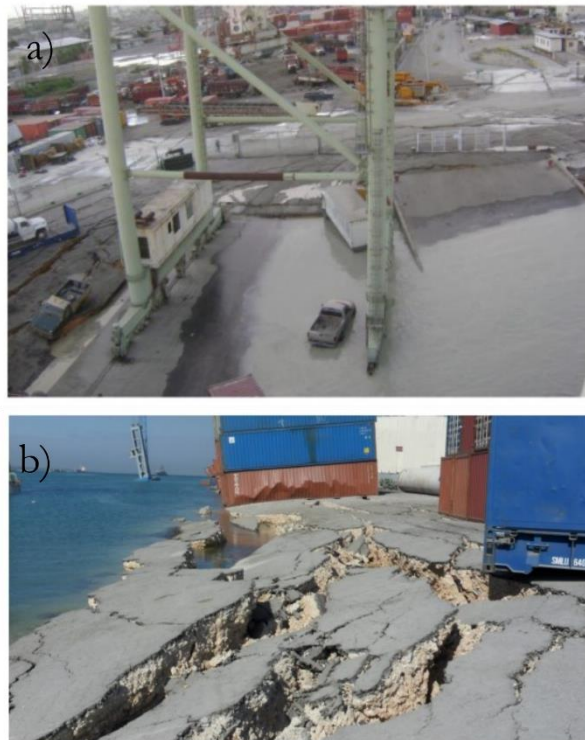
Figure 2.7. Lateral spreading damage to the North Wharf of the Port-au-Prince seaport after 2010 Haiti earthquake. Taken from Green et al. (2011).
