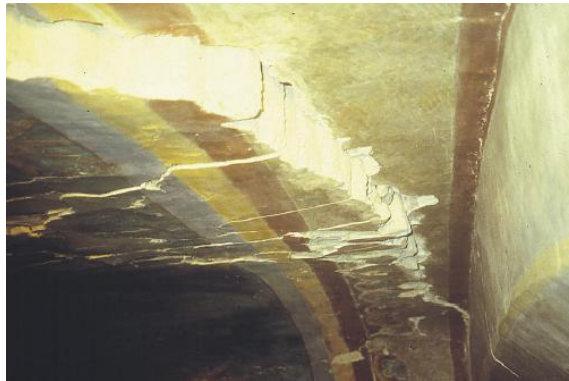
Figure 6.7 Cracks and deformations in the vaults with relative displacements till 30 cm (Croci, 2000)
