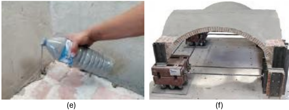
Figure 7.21 Application of the strengthening TRM system: (a) injecting fluid mortar GeoCalce antisismico FL in the cracks, (b) detail of the geosteel grid 200 embedded in GeoCalce antisismico F, (c) application process, (d) detail of the corners close to the infill with geosteel grid 600, (e) injecting the fluid mortar GeoCalce antisismico FL, (f) final appearance of the strengthened model (Bianchini et al., 2024)
