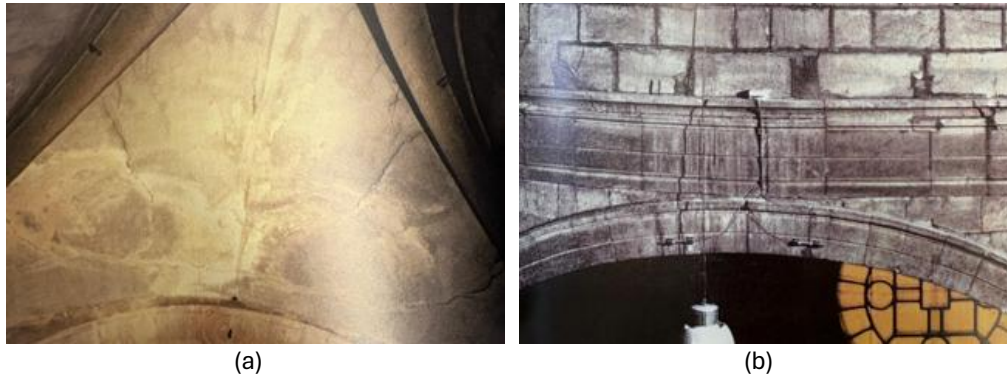
Figure 6.3 Cathedral of Pavia (Italy) cracking pattern on triangular vault adjacent to the central octagon (a) and on the major arch of the octagon (b) (Calvi & Palenzona, 2013)
