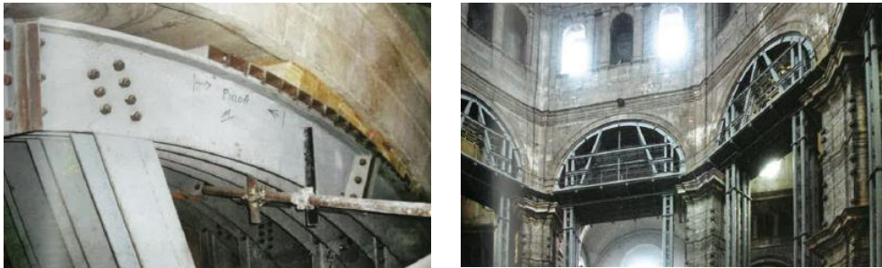
Figure 7.6 Centering and shoring frames used to support the arches bearing the octagonal drum (Cathedral of Pavia, Pavia – Italy)
