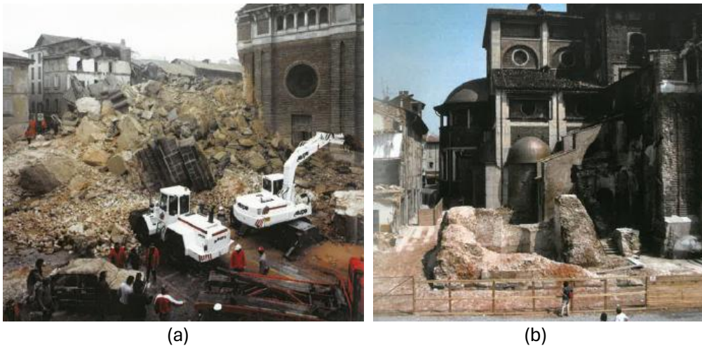
Figure 6.2 Cathedral of Pavia (Italy): debris-removal operations following the collapse of the Civic Tower (a), and base of the Civic Tower after the clearing operations (b) (Calvi & Palenzona, 2013)
