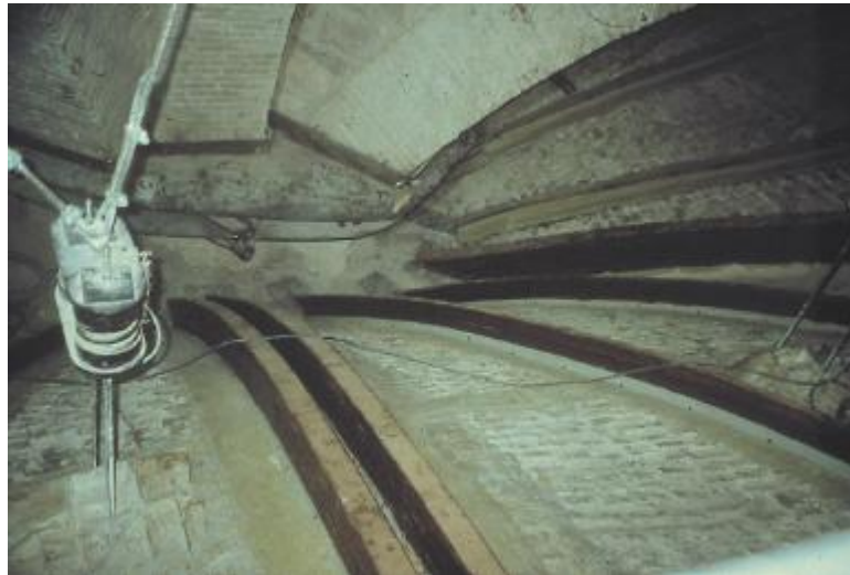
Figure 7.10 The new ribs, made of a central timber nucleus and external aramidic fibres. In the background, the steel belt to anchor the base of the arches which sustain the roof is visible (Croci, 2000)
