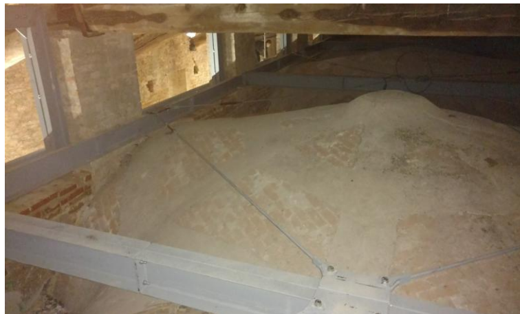
Figure 7.3 Example of perimetral steel frame (Santa Monica, Cremona – Italy, project by Studio Calvi)
